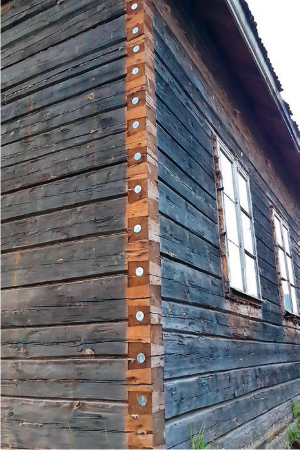
Hirsitalon laputettu nurkka | Patched up log house corner
